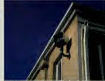
An infrared wireless link on the side of the building.
